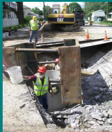
Photo: Emily Guerin / For The Forecaster Workers install new water mains, storm water drains and sewers along Washington Avenue in Portland,
